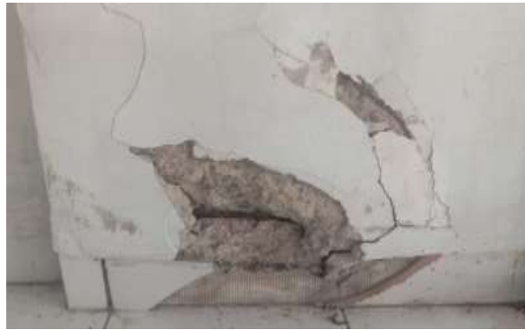
Figure 1. Severe Spalling and Cracking on First-Floor Column
