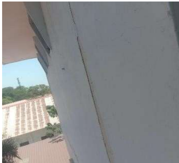
Figure 3. Minor Hairline Crack on Third-Floor Column
