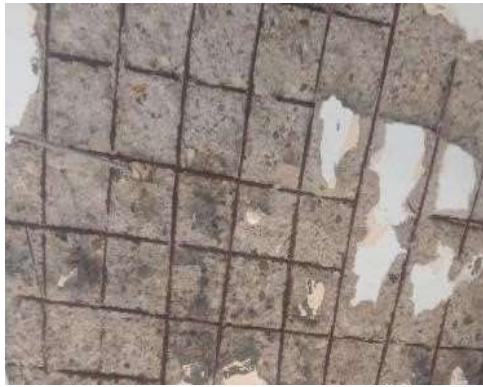
Figure 4. Severe Concrete Spalling and Reinforcement Exposure on First-Floor Slab
