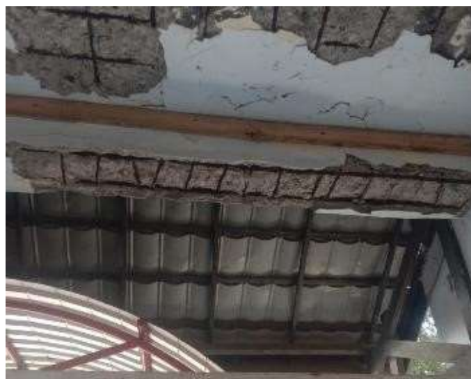
Figure 6. Extensive Spalling and Reinforcement Exposure on First-Floor Beam
