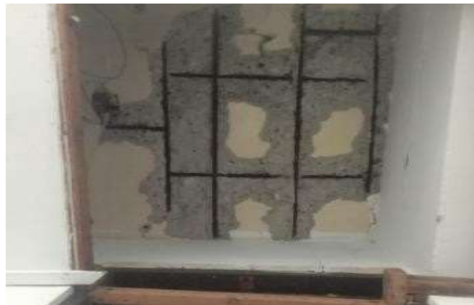
Figure 5. Localized Concrete Loss and Reinforcement Exposure on Second-Floor Slab
