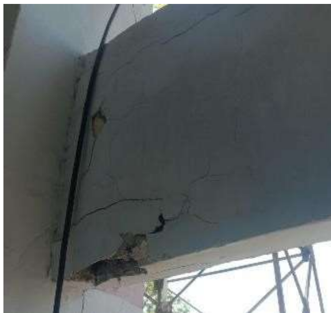
Figure 7. Cracking and Minor Concrete Loss on Second-Floor Beam
