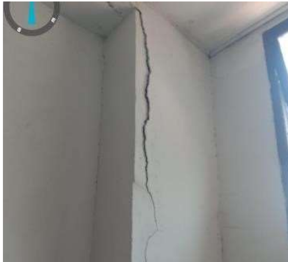
Figure 2. Vertical Cracking on Second-Floor Column
