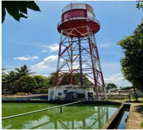
Figure 4. Water Tower' for Production and Hydrant
